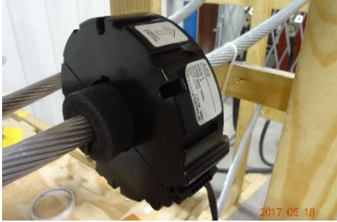
Figure 15. Picture of a final product of the submersible split-core sensor (RSS-1) installed in the test setup.
