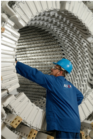
Figure 2. Stator end-winding of a turbo-generator
